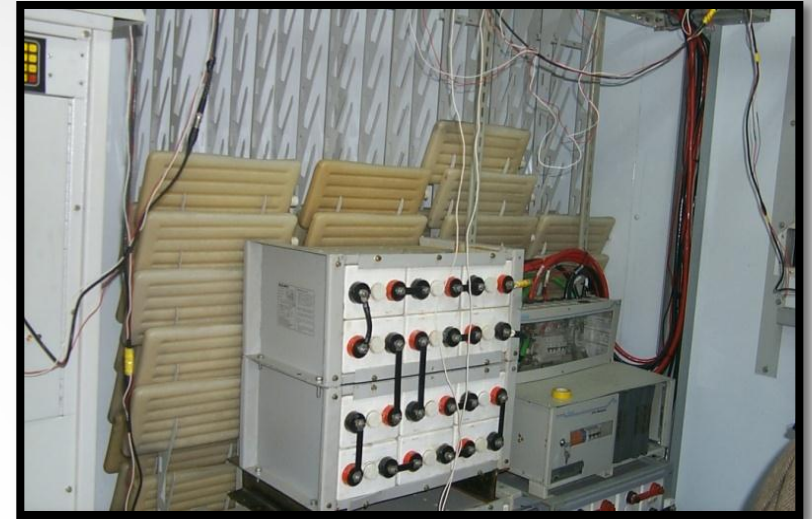
Telecom shelter optimization by using less power for temperature regulation
