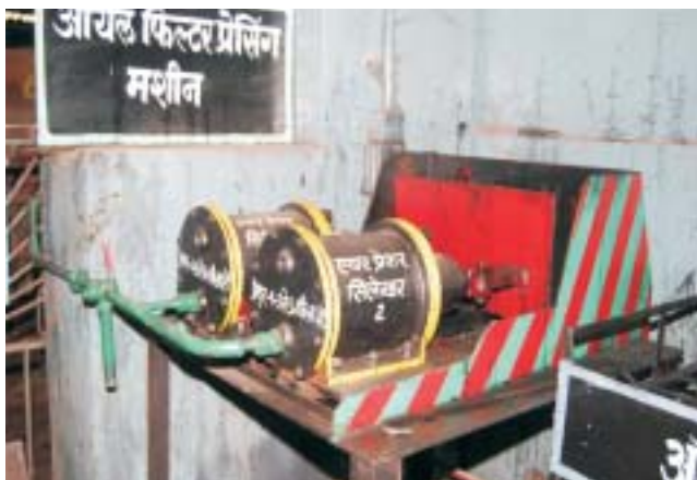
The oil filter press at Loco Repair Shop (LRS)
