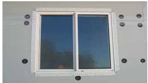
Photo 13. Panel joints with separate 150mm wide 160gsm fibreglass mesh strips applied directly over joints. (Only applicable to pre-rendered panels). All pre-rendered cladding panel joints to have reinforcing mesh applied over them as shown.
