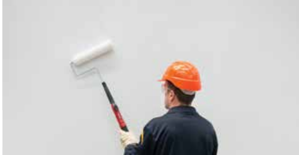
Photo 22. Application of primer coat onto finished rendered surface using a brush roller.
