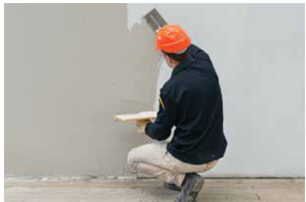
Photo 21. Application of final render coat. Total render thickness should be between 8mm and 10mm.
