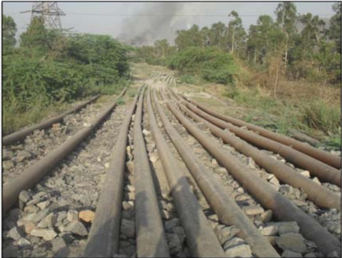
Figure 8 Pipelines from plant to the ash dyke
