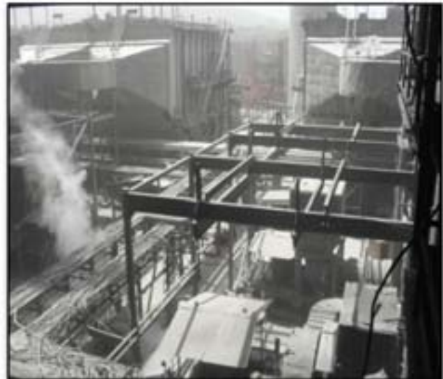
Figure 15 Boiler chamber of TPP
