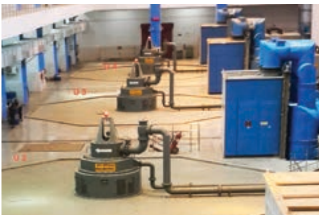
2 Units of 200 MW each of Koldam HEP commissioned by BHEL during the year
