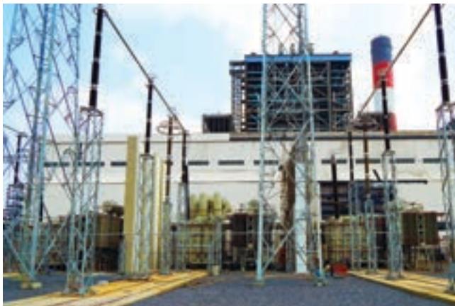
3x275 MVA 765 kV Transformer Bank, developed by BHEL, commissioned at Lalitpur 2
