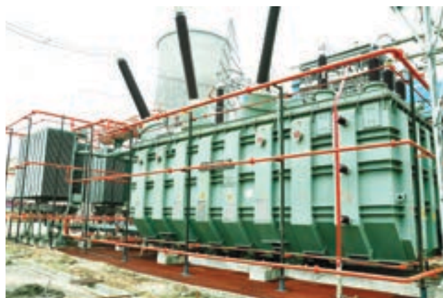
India's first 'Phase Shifting Transformer' at Kothagudem developed & manufactured by BHEL
