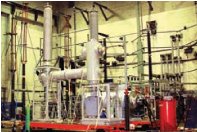
400 kV GIS indigenously developed and successfully type tested by BHEL
