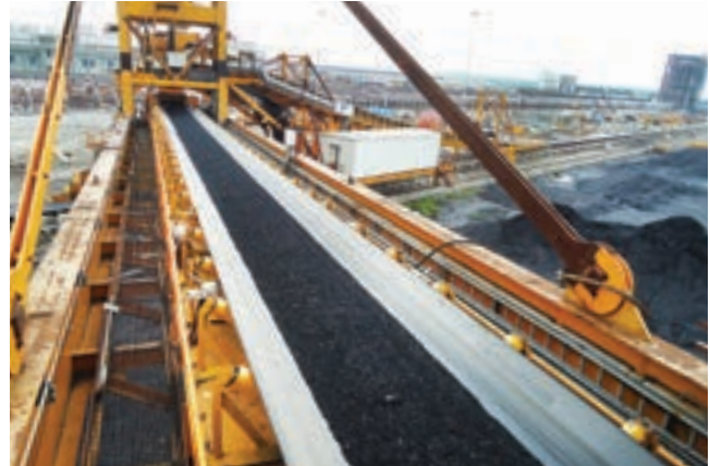
4000 TPH Stacker Reclaimer being fed by conveyor at NTECL, Vallur TPP
