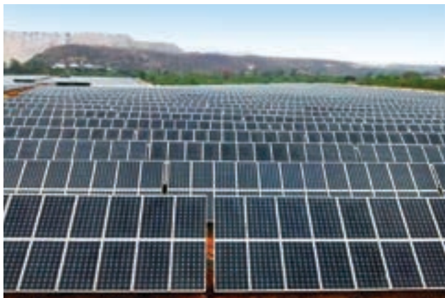
15 MW SPV Plant for NTPC Singrauli commissioned by BHEL
