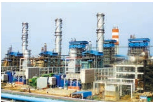
376 MW captive power plant set up by BHEL at IOCL's Paradip refinery
