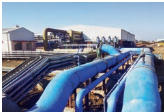
1000 cum/hr. treated water facility phase-1 commissioned at OPAL Raw Water Treatment Plant
