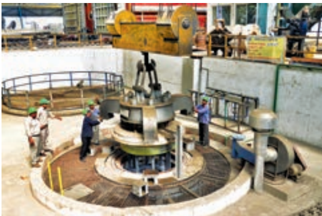
Vertical Shaft Furnace for heat treatment of more than 10M long forgings established at CFFP, Haridwar
