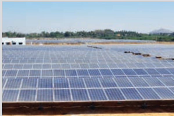
BAP Ranipet unit is the first unit of BHEL to install a 5 MWp grid interactive solar power plant
