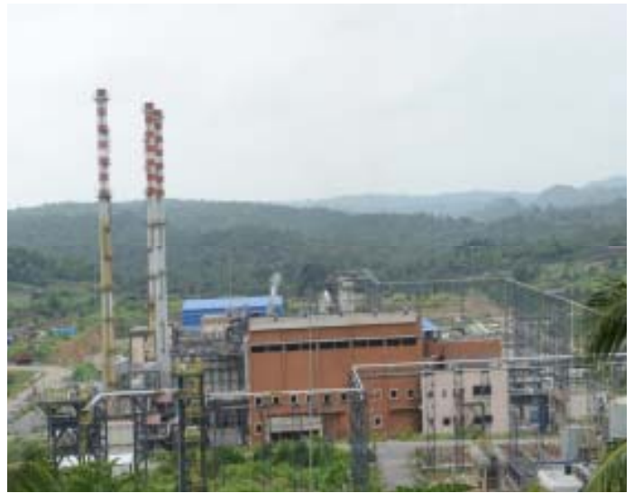
Captive Power Plant
