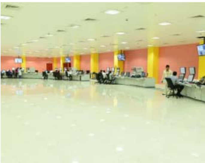
Master Control Room
